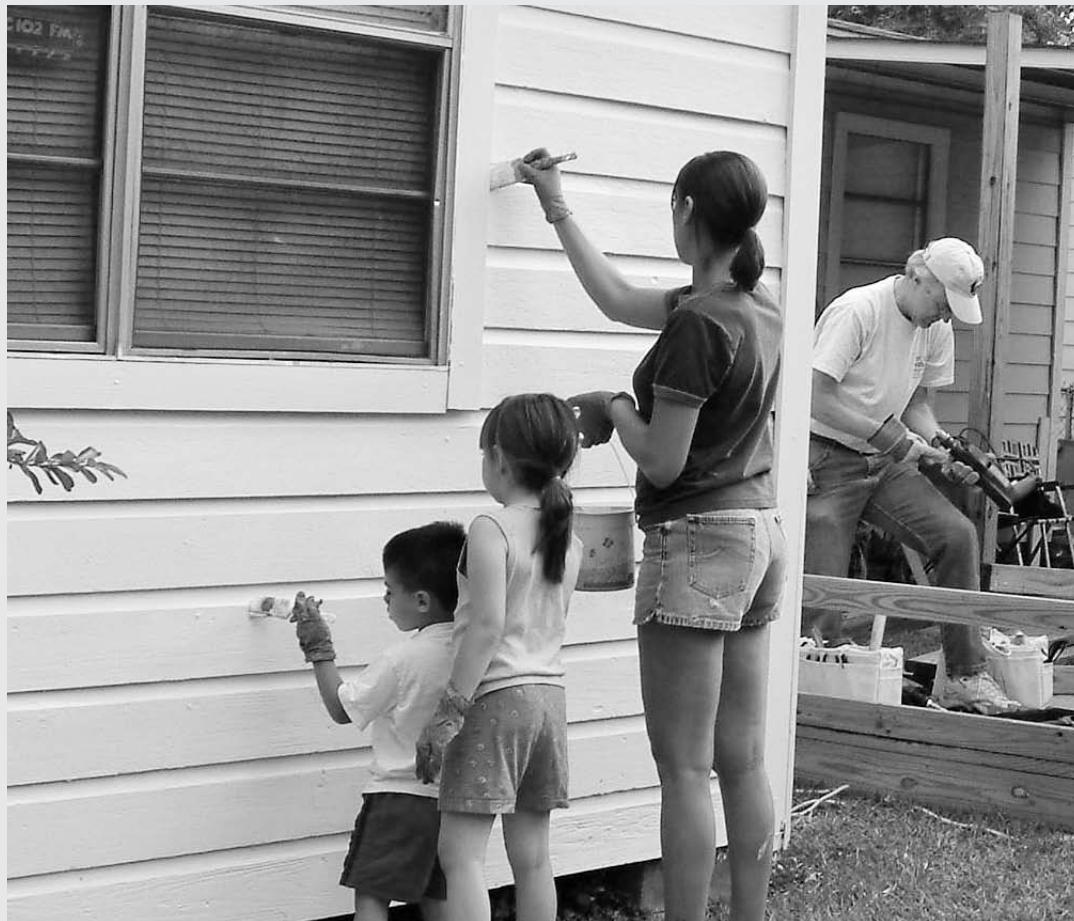
House Medics' volunteers of all ages work to repair the homes of low-income community elders. Photo courtesy of House Medics
